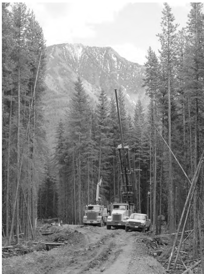
Figure 6: Geotechnical exploration drilling on the Bingay Creek coal property of Centermount Coal Limited.
