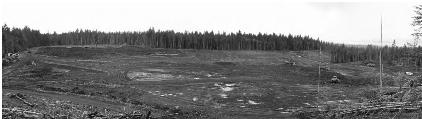
Figure 5: Site preparation of the 7 South area at Quinsam Mine, Vancouver Island. A coal seam is exposed in the centre of the frame.
